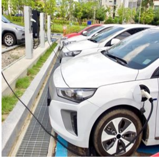
Public EV-Charging: City Lots
